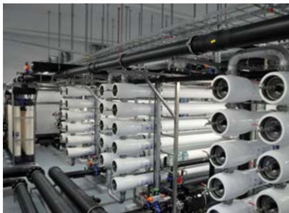
The Apateq water treatment plant treats brackish well water and pre-treated industrial process water.
